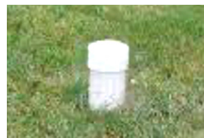
PROPERLY CAPPED SEWER CLEANOUT
