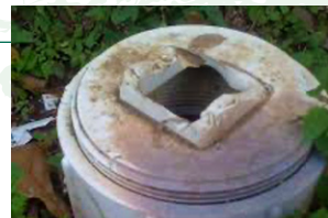
IMPROPERLY SEALED SEWER CLEANOUT
